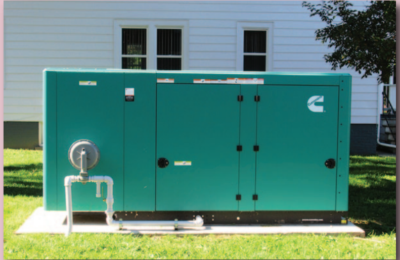
The generator purchased with the help of our donors in our 2019 Annual Appeal for the Sisters' Emergency and Safety Plan
